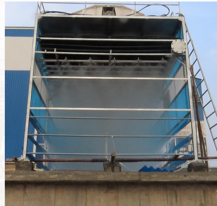
Induced Draft Mist Cooling Tower with-out any FILLS
