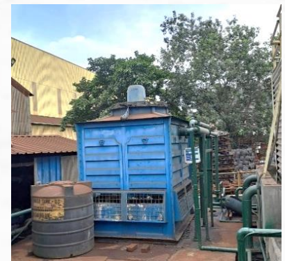
old cooling towers at M/s. RKFL
